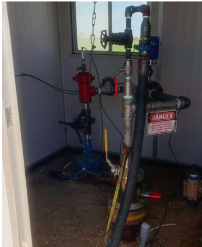
(a) Test setup showing the fluid withdrawal access point
