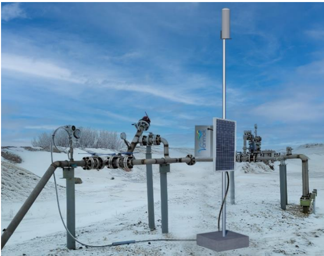
Figure 4 Typical installation of IoT Gateway connected to a pressure transmitter.
